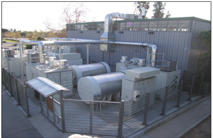
Figure 18. Fuel Cell installation
