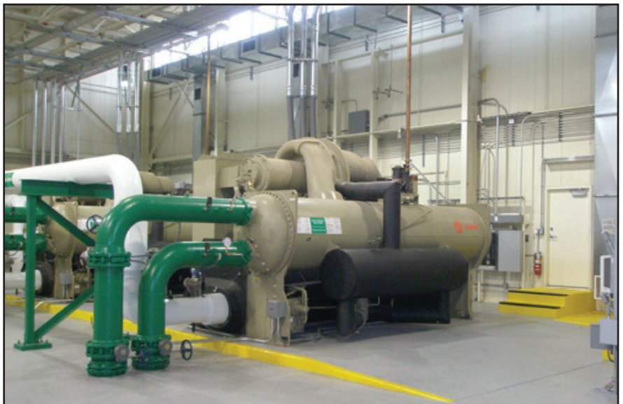
Figure 19. Inside chiller plant facility adjacent to fuel cells.
