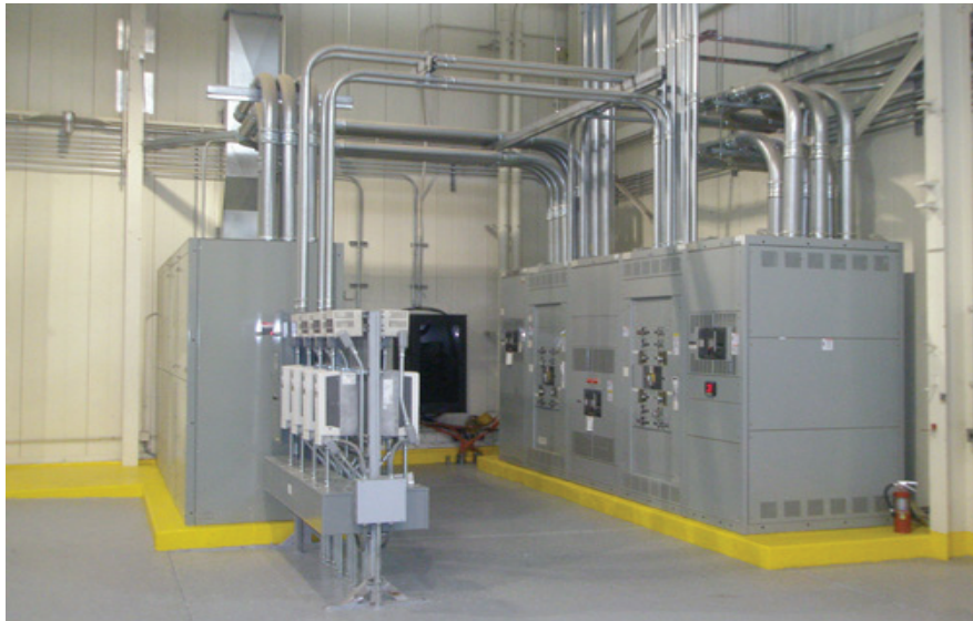
Figure 20. Rainforest controls inside chiller plant adjacent to fuel cells.
