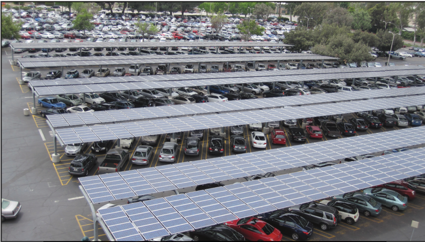
Figure 28. Second PV array at California State University, Northridge. Installed in parking lot B2.
